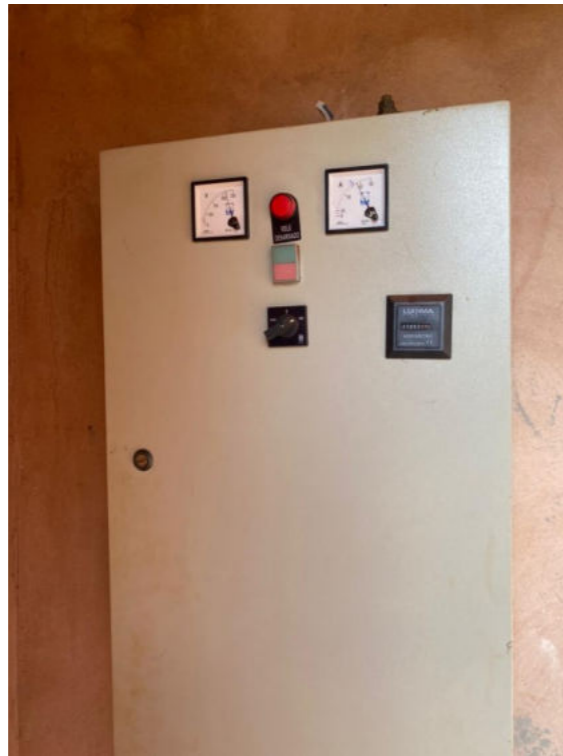
Figura 66 – Painel de controle.
